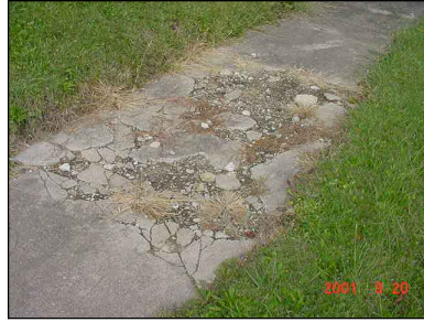
ANY SIDEWALK THAT IS DETERIORATED OR SHOWS SURFACE SPALLING, LEAVING IT VERY ROUGH, UNSAFE, OR WITH AGGREGATE PROTRUDING.
