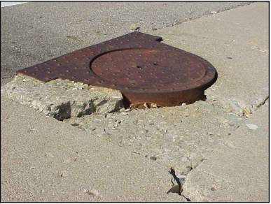
METAL OR OTHER PLATES, COVERS, OR GRATINGS THAT ARE NOT FLUSH (1/2 INCH OR MORE VERTICAL DIFFERENCE) WITH THE ADJOINING SIDEWALK SURFACE, ARE STRUCTURALLY UNSAFE, OR CAUSE A NUISANCE DUE TO SLIPPERY SURFACES ETC.
